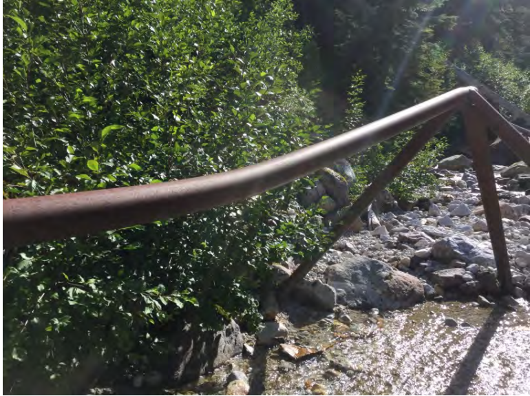
Trash rack damage struck by
