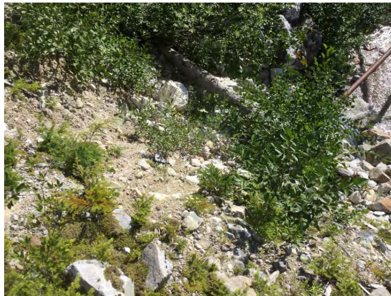
Fill slope upstream erosion at inlet
